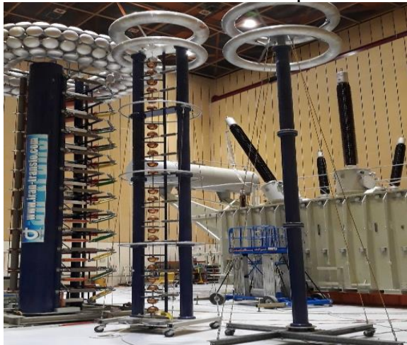
Fig. 6. The routine LI FAT setup on the 230/63/20 kV, 160 MVA power transformer at the HV test Lab
